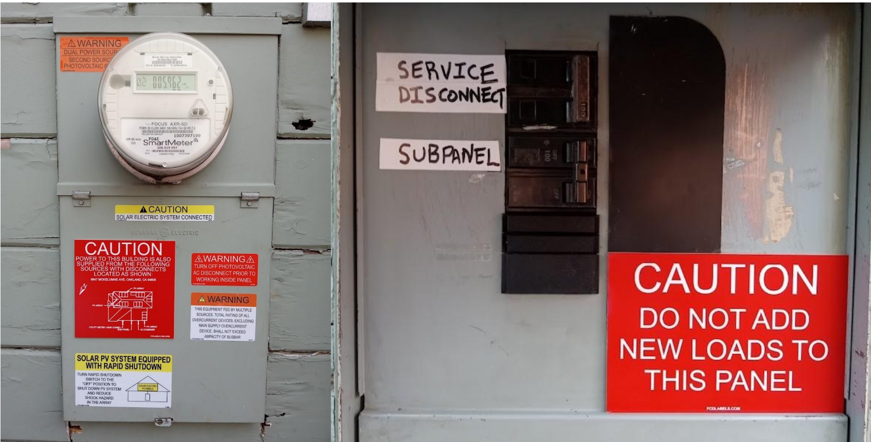
Existing main panel
