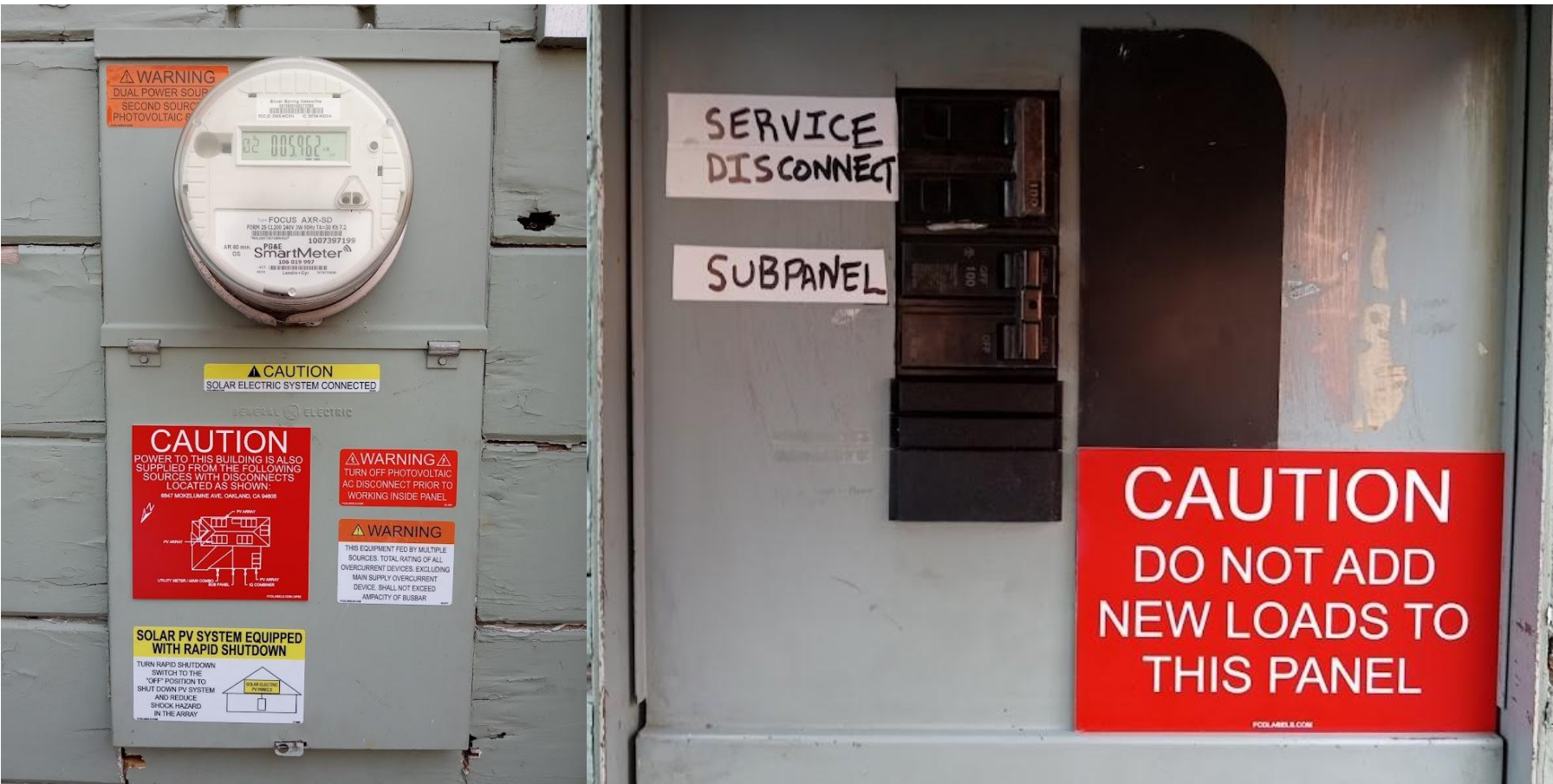
Existing main panel
